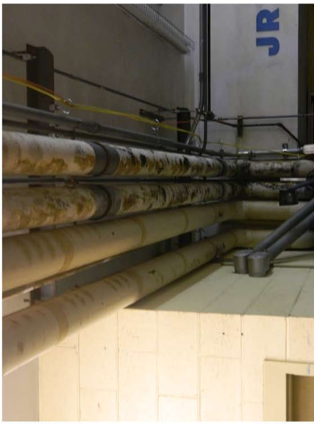
Deteriorated pipe insulation form water issues.
