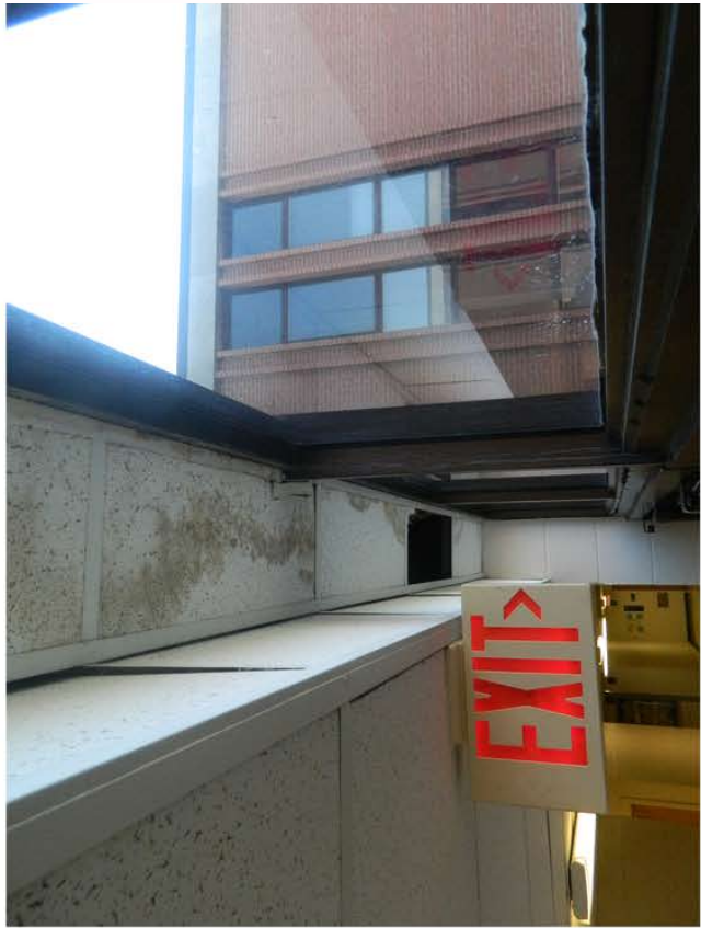
Water infiltration at exterior glazing
