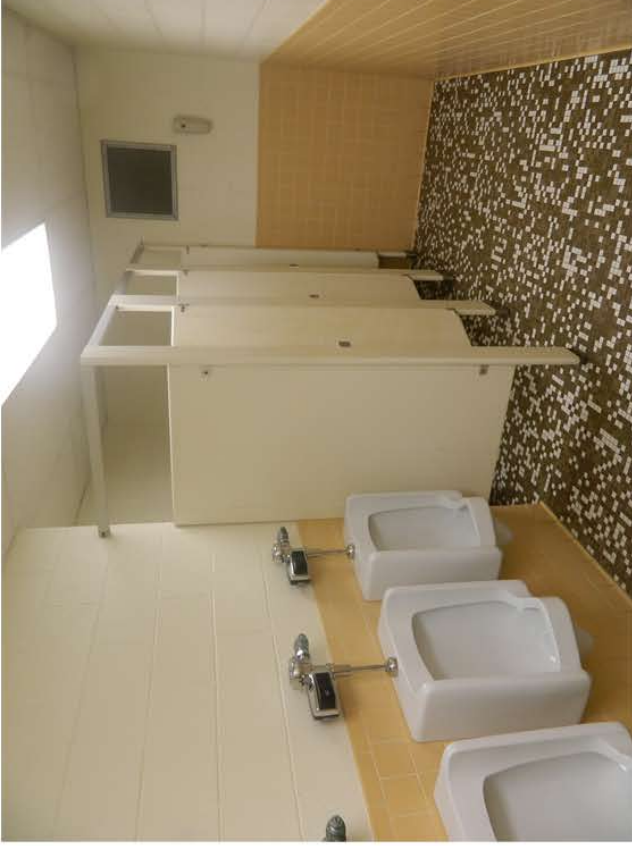
Non-ADA Compliant Restrooms
