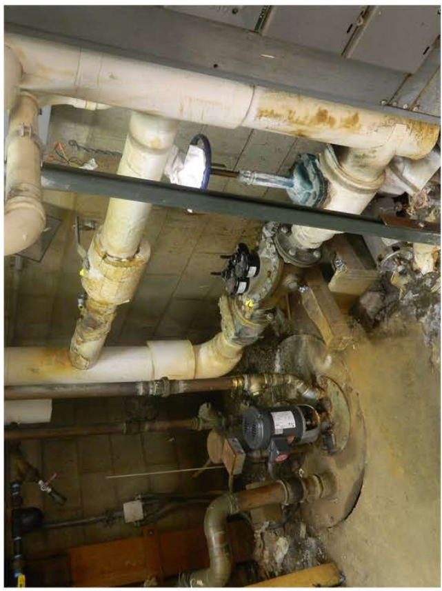
Deteriorated and aged piping.
