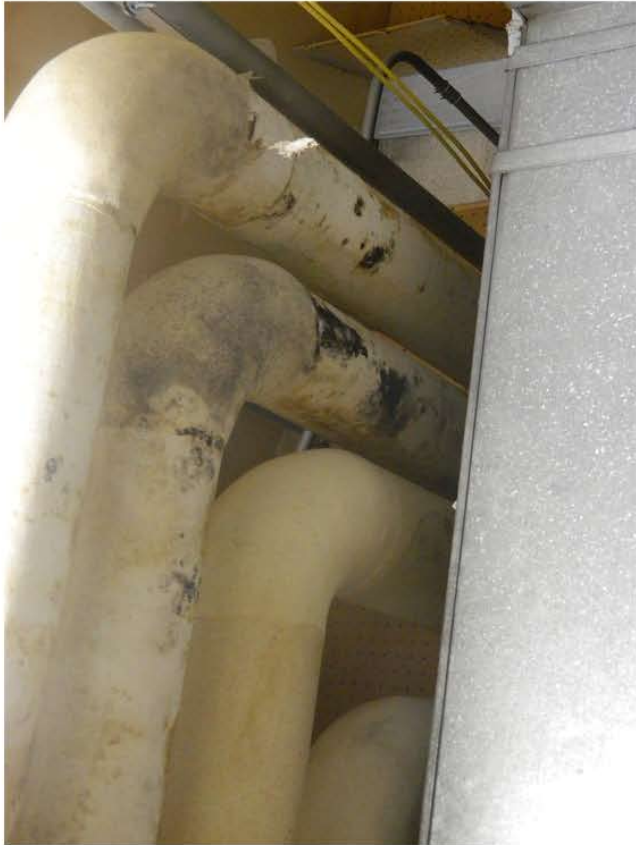
Deteriorated pipe insulation form water issues.
