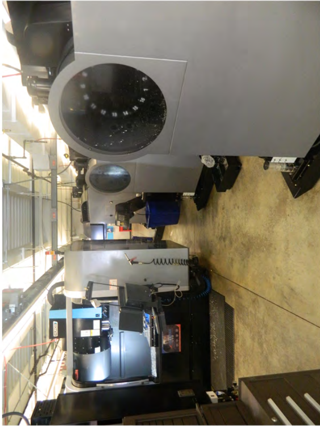
Machines spacing does not allow proper circulation space.
