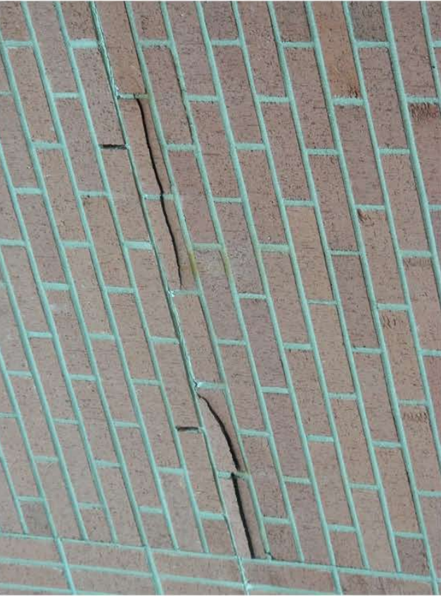
Exterior brick damage caused by flashing deterioration.
