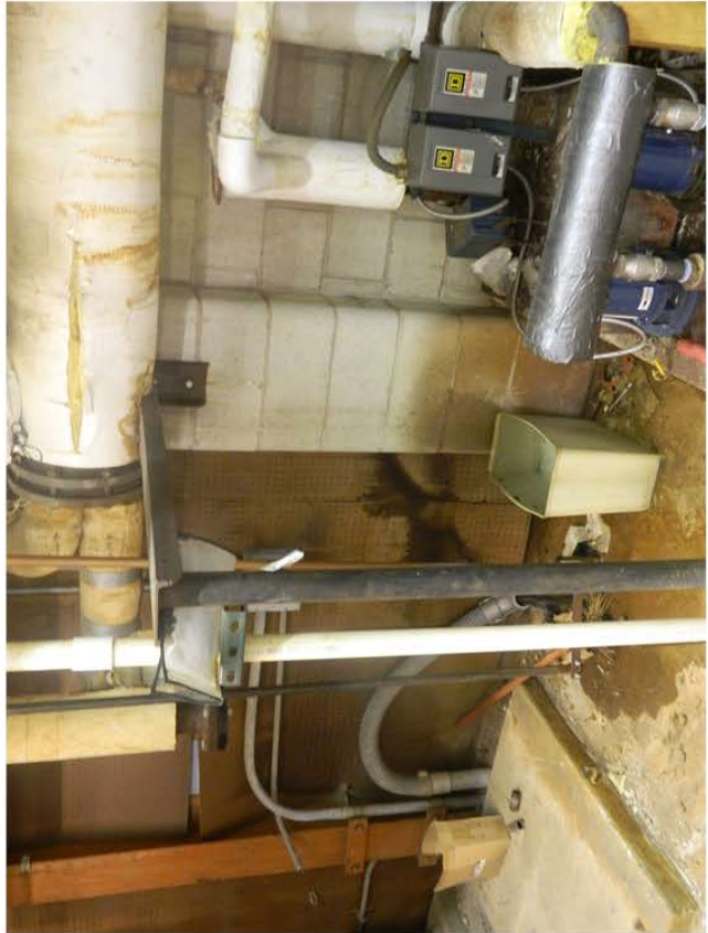
Active leaks in mechanical equipment.
