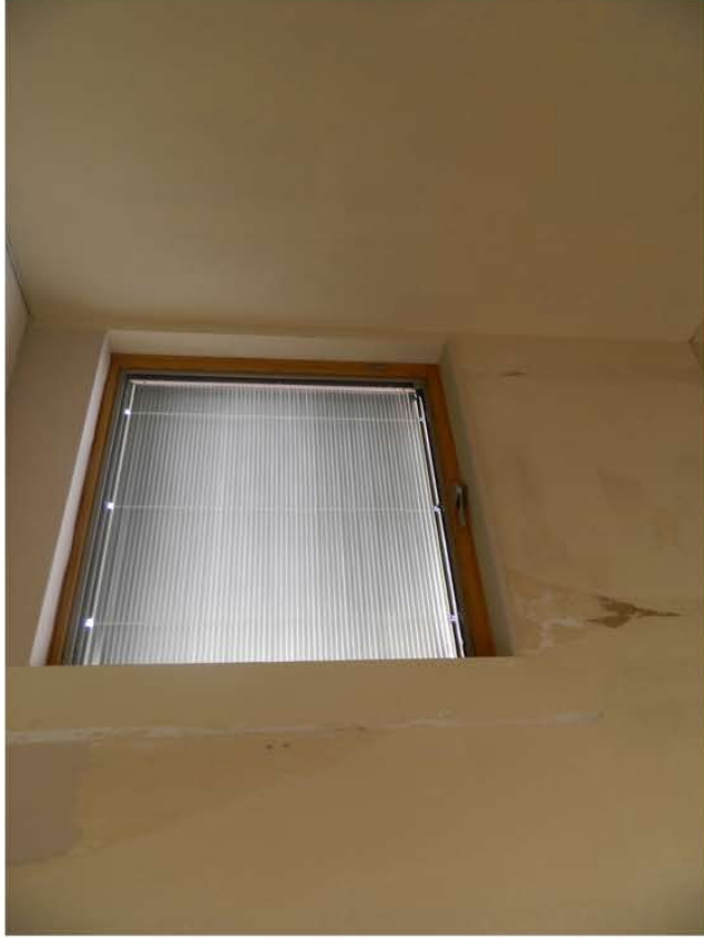
Damage at window location.
